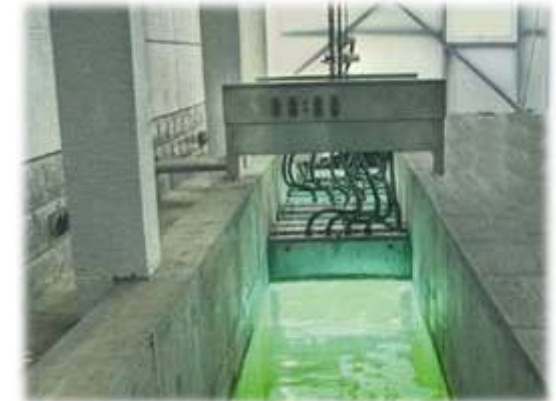
WWTP, Beijing China - 60,000 m 3 /day
