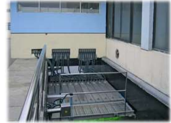
WWTP, Suzhou, China - 260,000 m 3 /day
