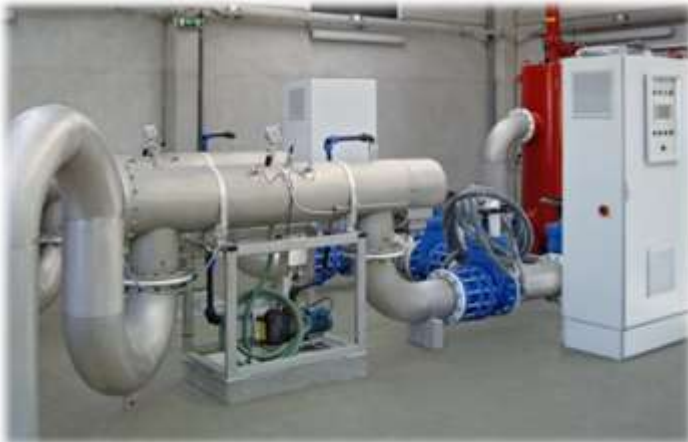
WWTP, Sesimbra, Portugal - 6,400 m 3 /day
