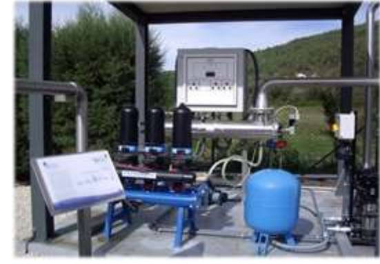
Municipal WWTP, Portugal, 480 m 3 /day
