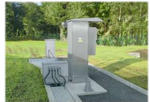
WWTP, Chateaulin, France - 8,400 m 3 /day
