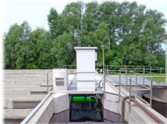
WWTP, Pecs, Hungary - 86,400 m 3 /day
