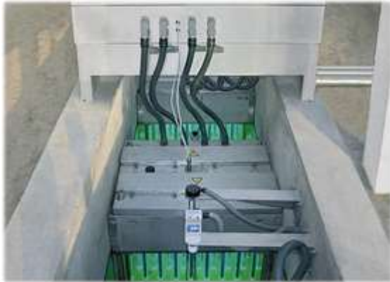
WWTP, Gadong, Brunei -58,200 m 3 /day
