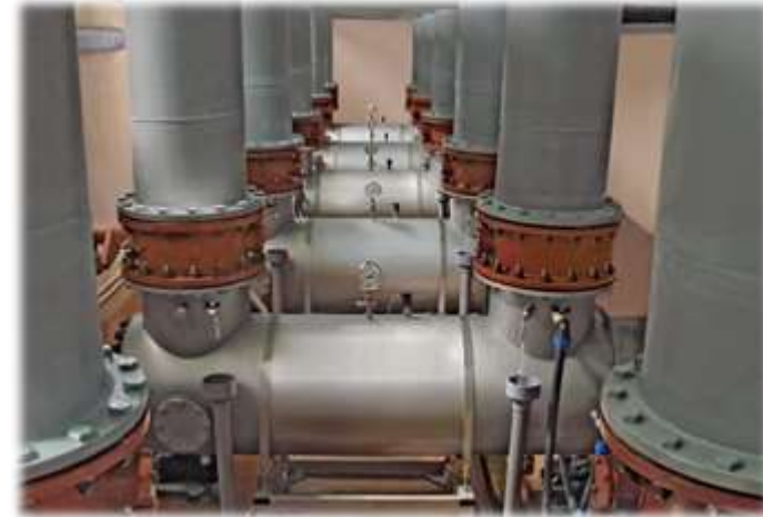
WWTP, De-Friz , Vladivostok, Russia - 18,000 m 3 /day
