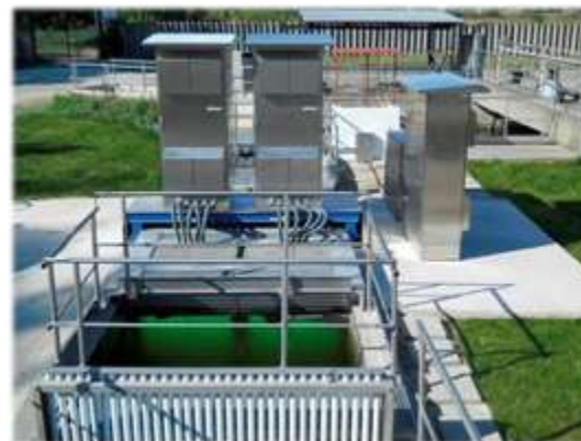
South WWTP, Budapest, Hungary - 80,000 m 3 /day
