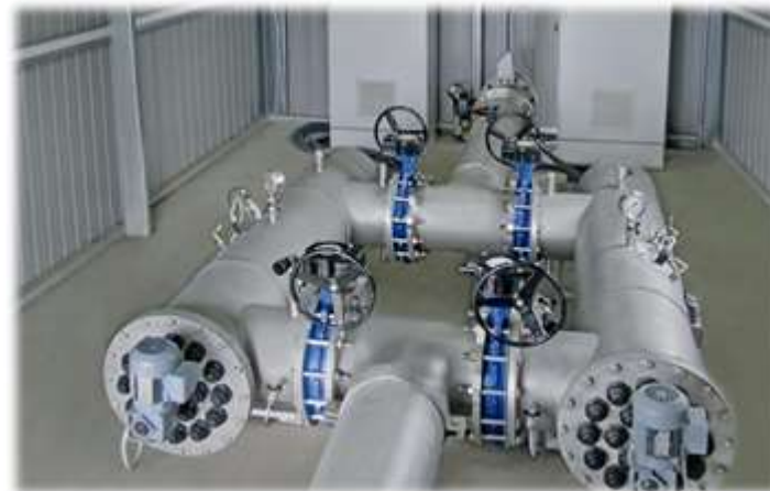
WWTP, Port Fairy, Australia - 6,100 m 3 /day
