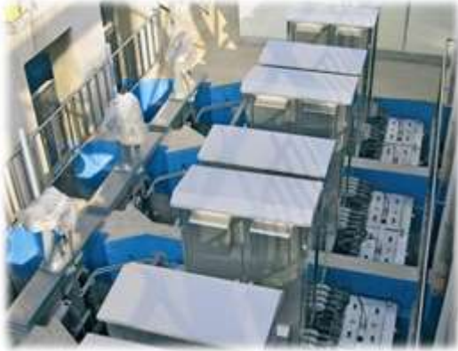
WWTP, Gumi, South Korea - 330,000 m 3 /day
