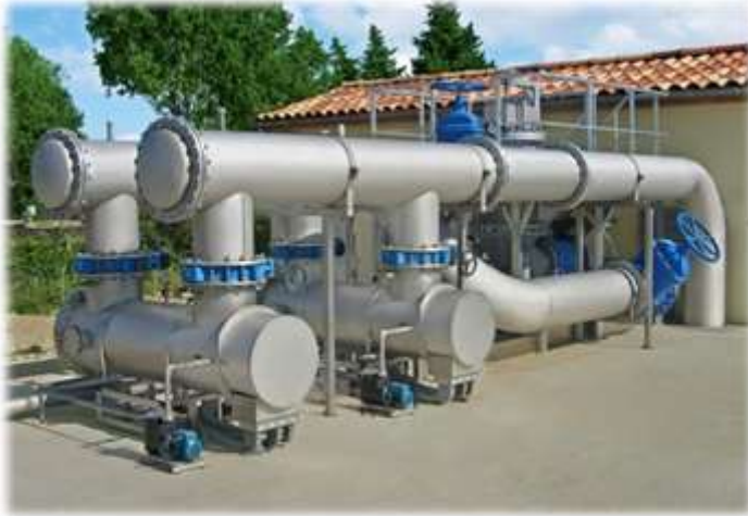
WWTP, Orange, France - 36,000 m 3 /day
