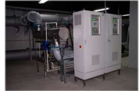
Drinking water, Poland 16,800m 3 /day
