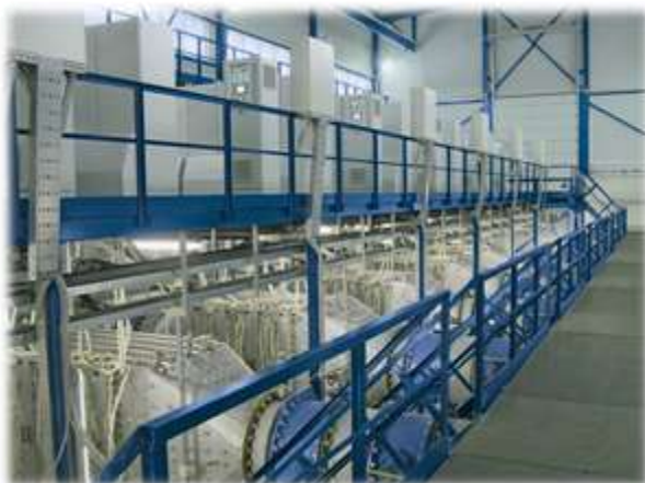
North WTP 1,584,000 m 3 /day
